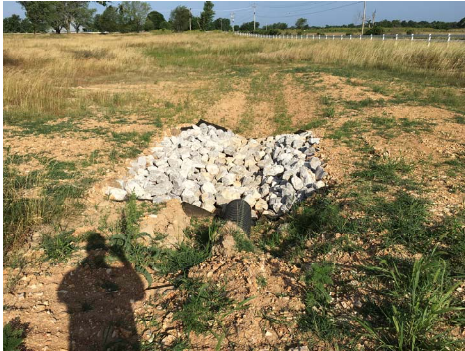
Photo 9 – Outfall 12” pipe with outlet riprap apron
