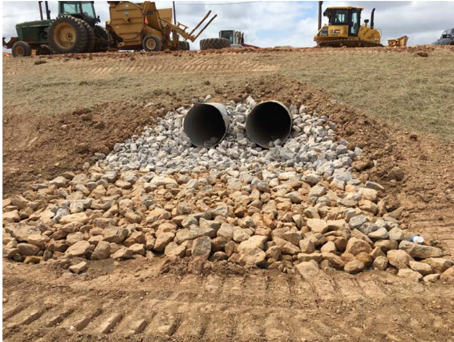
Photo 11 – Sedimentation Basin Inlet: Dual 42” CMP with RipRap Apron
